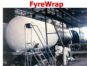
Tank Car Insulation
