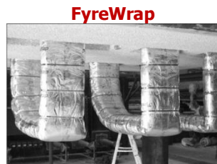
Cable Tray Insulation
